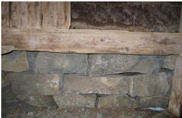
At the bottom of the wall at Reynistaður is a dry-stone base ( þurrt grjót ). Right: a corner-post stands on a foundation stone. The sill beam stands free of the ground. The ends of the wall boards are slotted into the beam.
