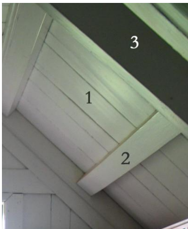
Right. 1 Roof clad with boards laid across from ridge to wall ( reisifiöl ). 2 Purlin. 3 Part of raft ( sperra ).
