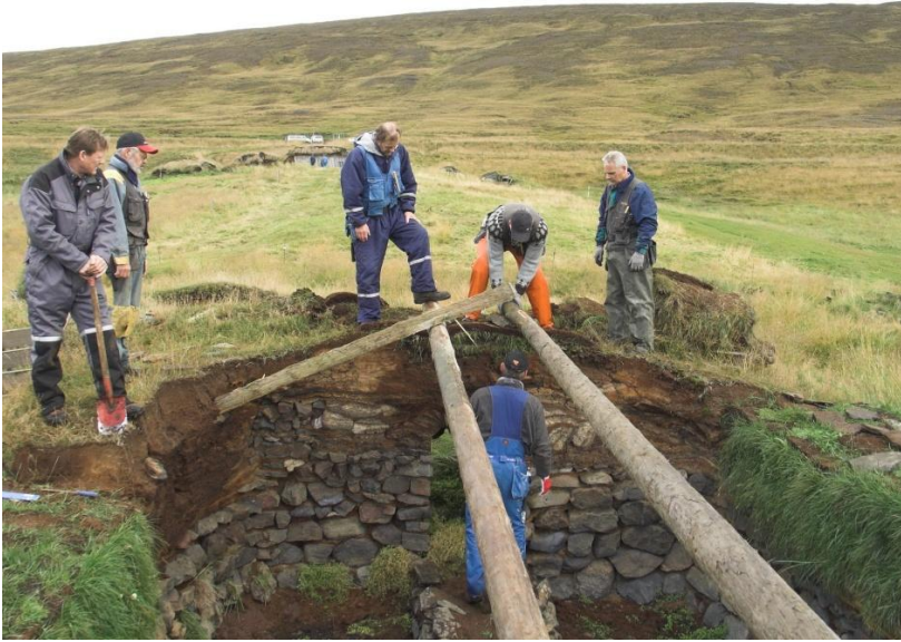
Tyrfingsstaðir. Twin-beam roof: the beams have been laid, and the first rafter is being put in place. The rafter lies on a small slab atop the wall.
